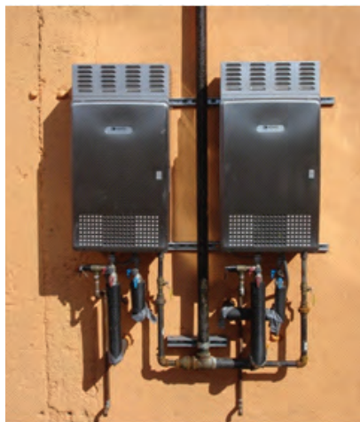
Two NC380-SV-ASME installed outside of the restaurant.
