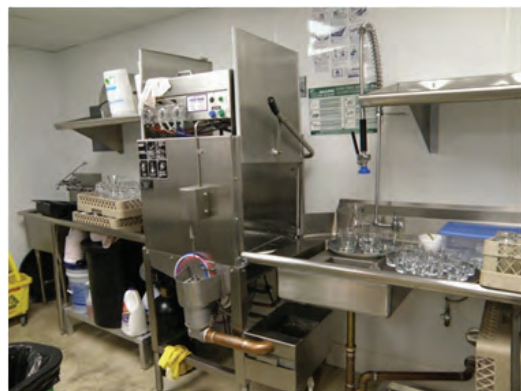
One of two commercial dishwashers in the restaurant requiring 4 GPM each @ 160-degree F.
