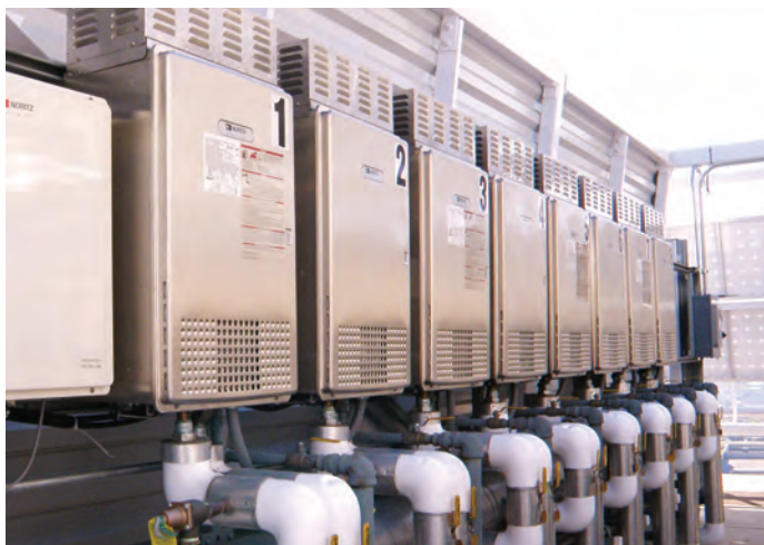
Eight Noritz N-1321M-ASME commercial water heaters on the roof top for 208 guest rooms.
