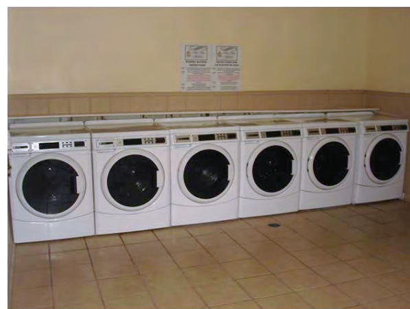
Laundry Room with 6 washing machines.
