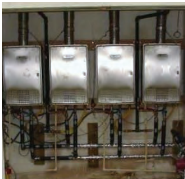
Four NC380-SV-ASME installed in Mechanical Room, previously occupied by two 100 gal. tank units.
